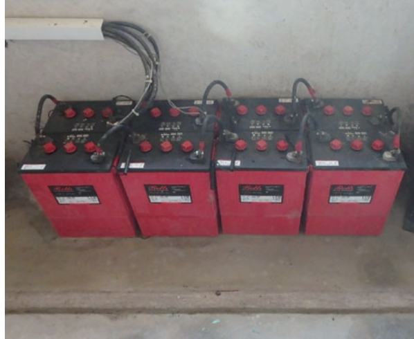
Fig. 8.4 A 48 V battery bank for a mini-grid in Kenya consisting of a string of eight, six-volt batteries arranged in series (courtesy of author)
