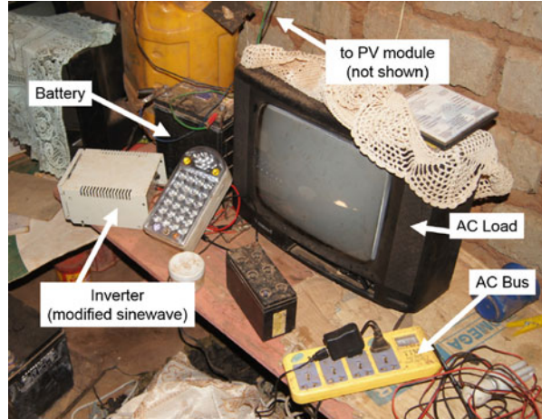
Fig. 9.1 This improvised solar-powered system has no controllers (courtesy of author)
