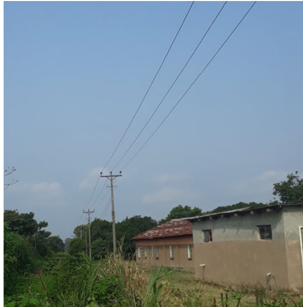
Fig. 3.4 A typical three-phase overhead distribution line (courtesy of R. Ngoma)
