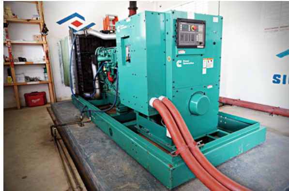
Fig. 5.11 A 660 kW diesel gen set used to power a mini-grid in Haiti (courtesy of Sigora Haiti)
