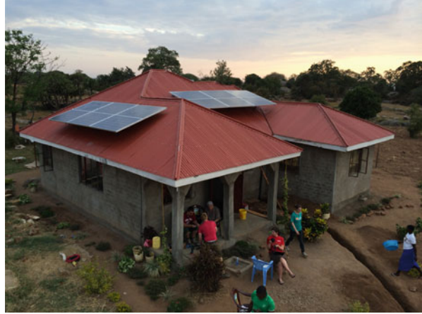
Fig. 7.1 A 3 kW PV array split into two strings in Kenya (courtesy E. Patten)
