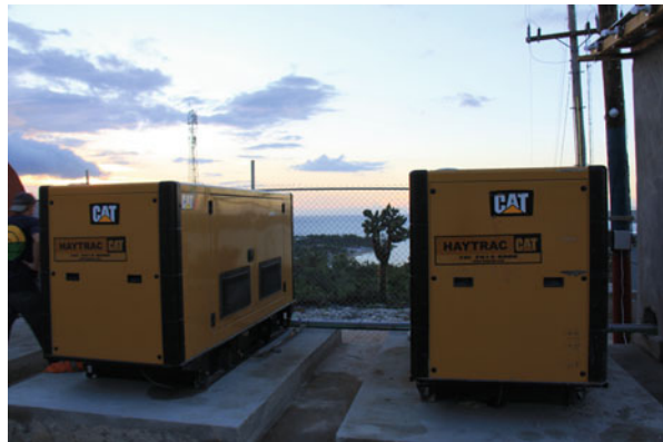
Fig. 12.21 Two 100 kW gen sets used in the Môle-Saint-Nicolas mini-grid (courtesy of Sigora Haiti)
