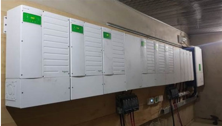
Fig. 9.3 The control room of a large mini-grid in Nigeria, consisting of inverters, charge controllers, and system monitoring equipment (courtesy of GVE Projects)
