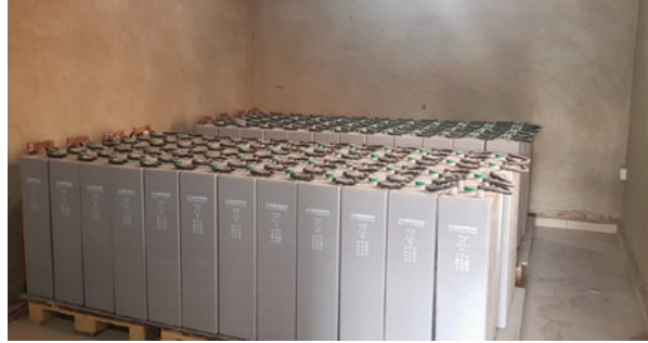
Fig. 8.21 Battery bank from a mini-grid in Nigeria; the battery bank has not been connected to the DC bus (courtesy of GVE Projects)
