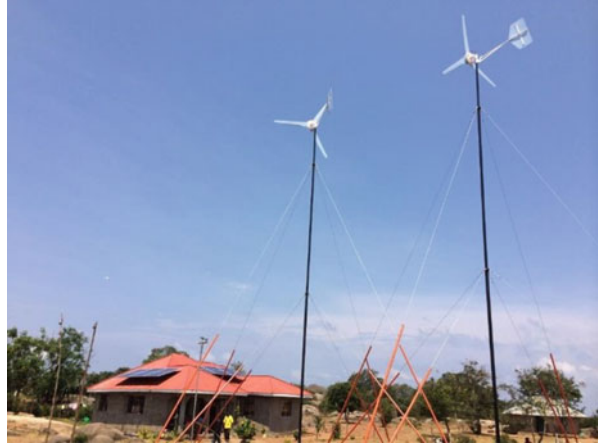
Fig. 4.2 A small-scale, decentralized, hybrid mini-grid using wind and solar power in Muhuru Bay, Kenya (courtesy E. Patten)
