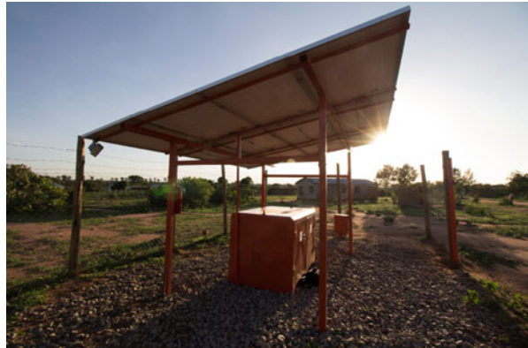
Fig. 12.24 The PV array of the Ighombwe mini-grid with the batteries, inverters and meters securely located in the housing below (courtesy of PowerGen)
