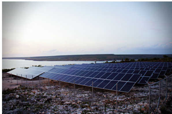
Fig. 12.22 A 200 kW PV array is used in the Môle-Saint-Nicolas mini-grid (courtesy of Sigora Haiti)
