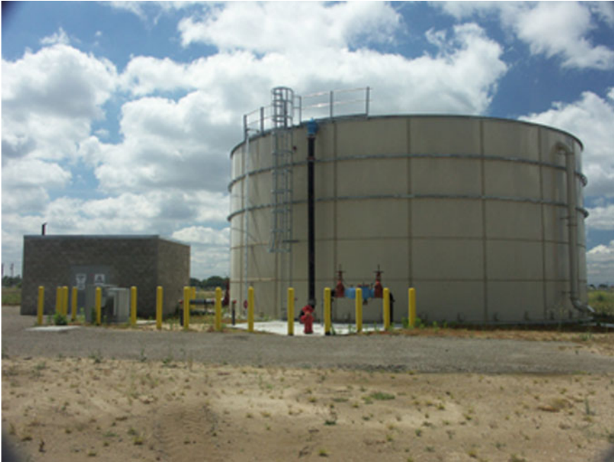
Fig. 5.2 A typical fire fighting water storage tank
