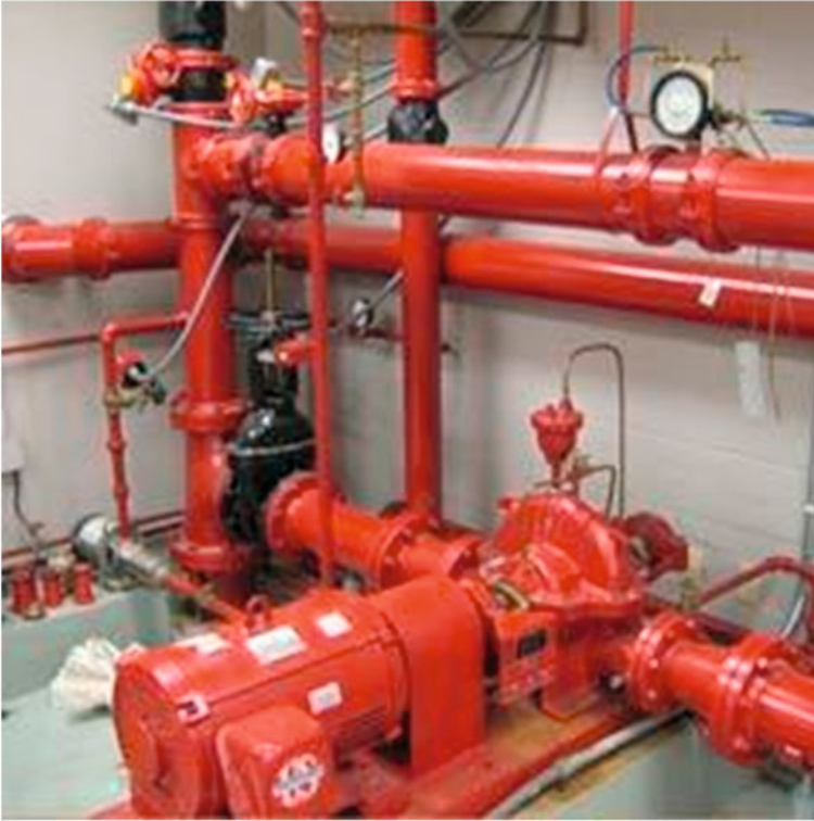
Fig. 5.1 A fire pump installation
