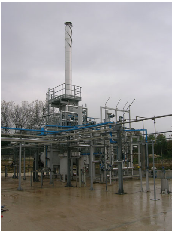
Semi-industrial membrane-based steam reformer installed in Chieti Scalo (Italy)
