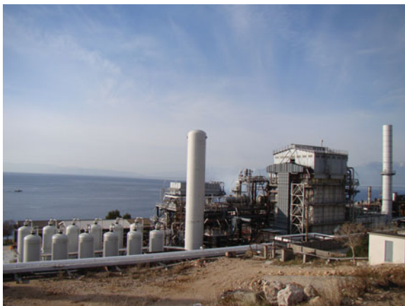
Fig. 5.6 NG tubular fired steam reforming plant (Courtesy from Tecnimont-KT)
