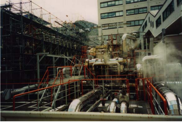
Fig. 5.4 Operating plant, Ohi, Japan
