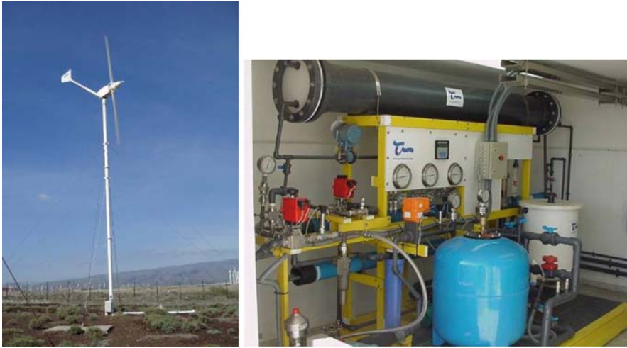
Fig. 10.7 The ITC wind/RO system in the Canary Islands
