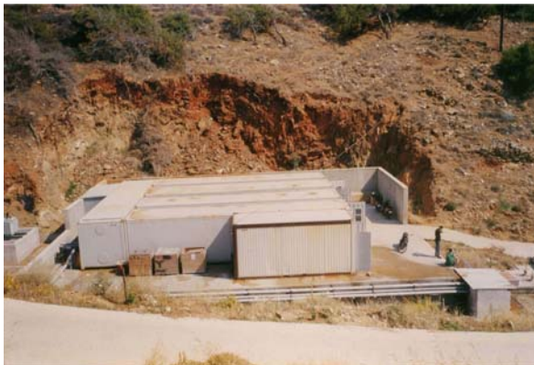
Fig. 9.30 View of the RO plant on the Island of Syros Source: [31]
