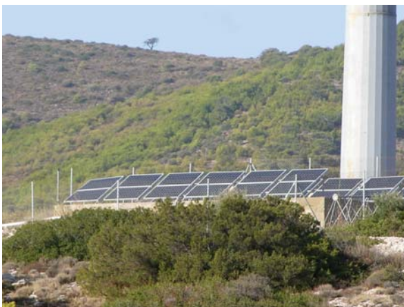
Fig. 9.26 CRES 4 kWp PV unit
