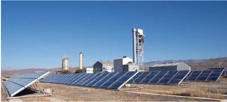
Fig.10.1 The solar thermal field of the solar MED plant in Almeria
