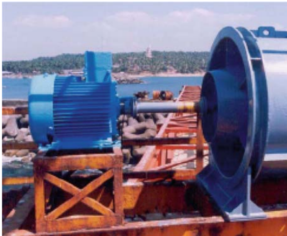
Fig. 9.32 View of the alternator, Vizhinjam plant
