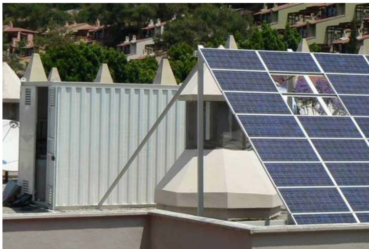
Fig. 10.6 The PV/RO system in Turkey
