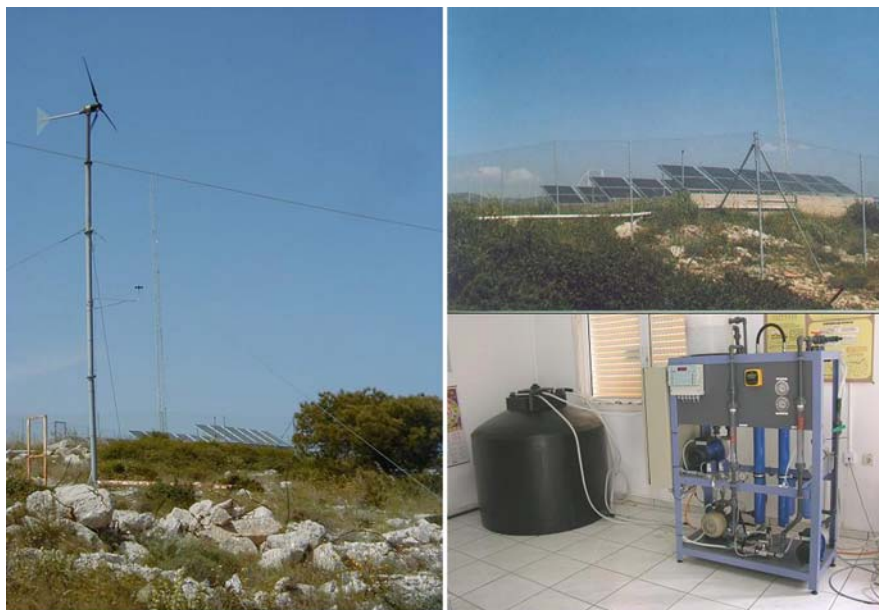
Fig. 10.9 The hybrid RO system installed in Lavrio by the centre for renewable energy sources
