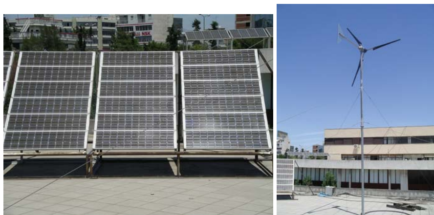
Fig. 10.8 The hybrid energy system that powers the RO at the Agricultural University of Athens
