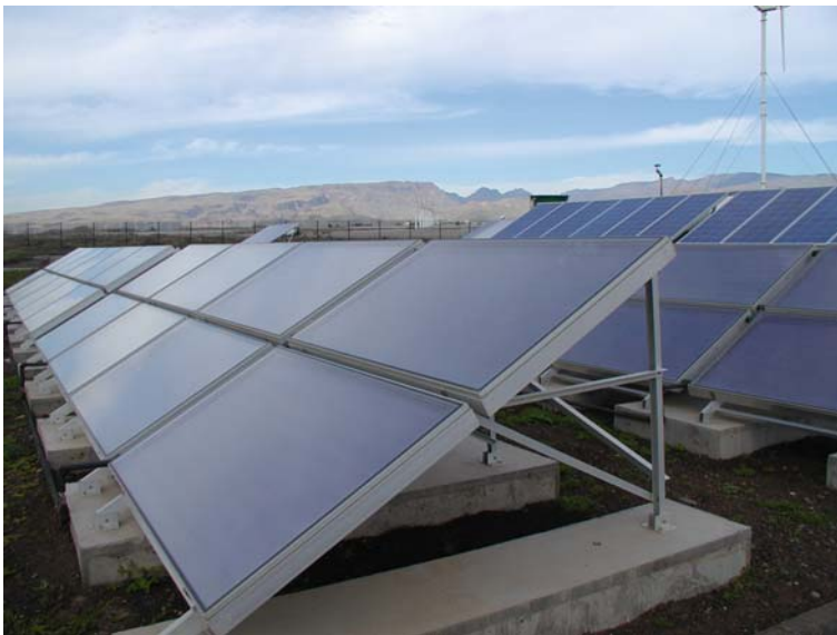
Fig. 10.4 The solar collector system of the 1 m 3 /day MD plant
