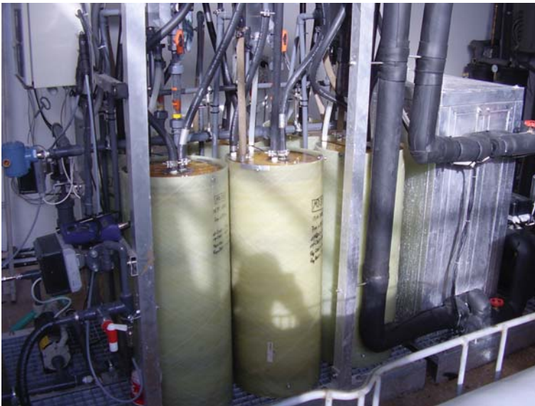
Fig. 7.14 Desalination unit with five MD modules and heat exchanger (on the right)
