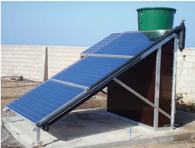
Fig. 7.10 Compact system installed in December 2007 in Tenerife, Spain
